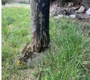
Figure 7.0 - Base of timber column with evidence of rot
