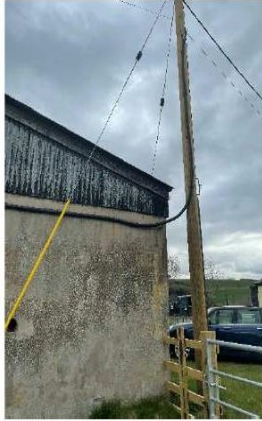
Figure 5.0 - Telegraph pole at SW corner of the barn
