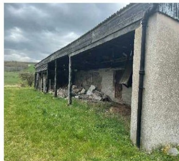
Figure 6.0 - North elevation of the Black Barn with partial access to the inside of the barn
